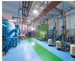
100% of the wastewater treated and reused onsite
