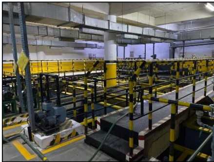
View of STP Room Tower 8, 9, 10
