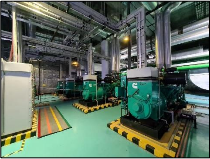
View of DG Room
